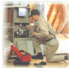
Regular maintenance on your heating system will help keep repairs & breakdowns to a minimum.
